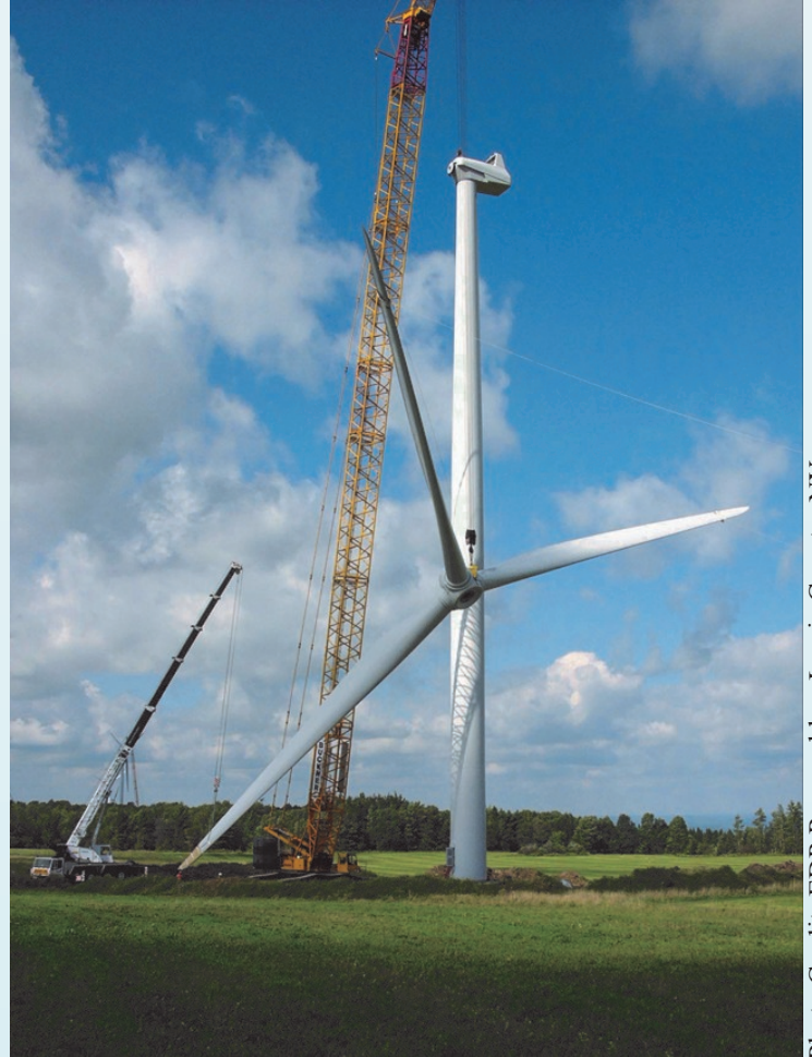
Photo Credit: EDP Renewables. Lewis County, NY
