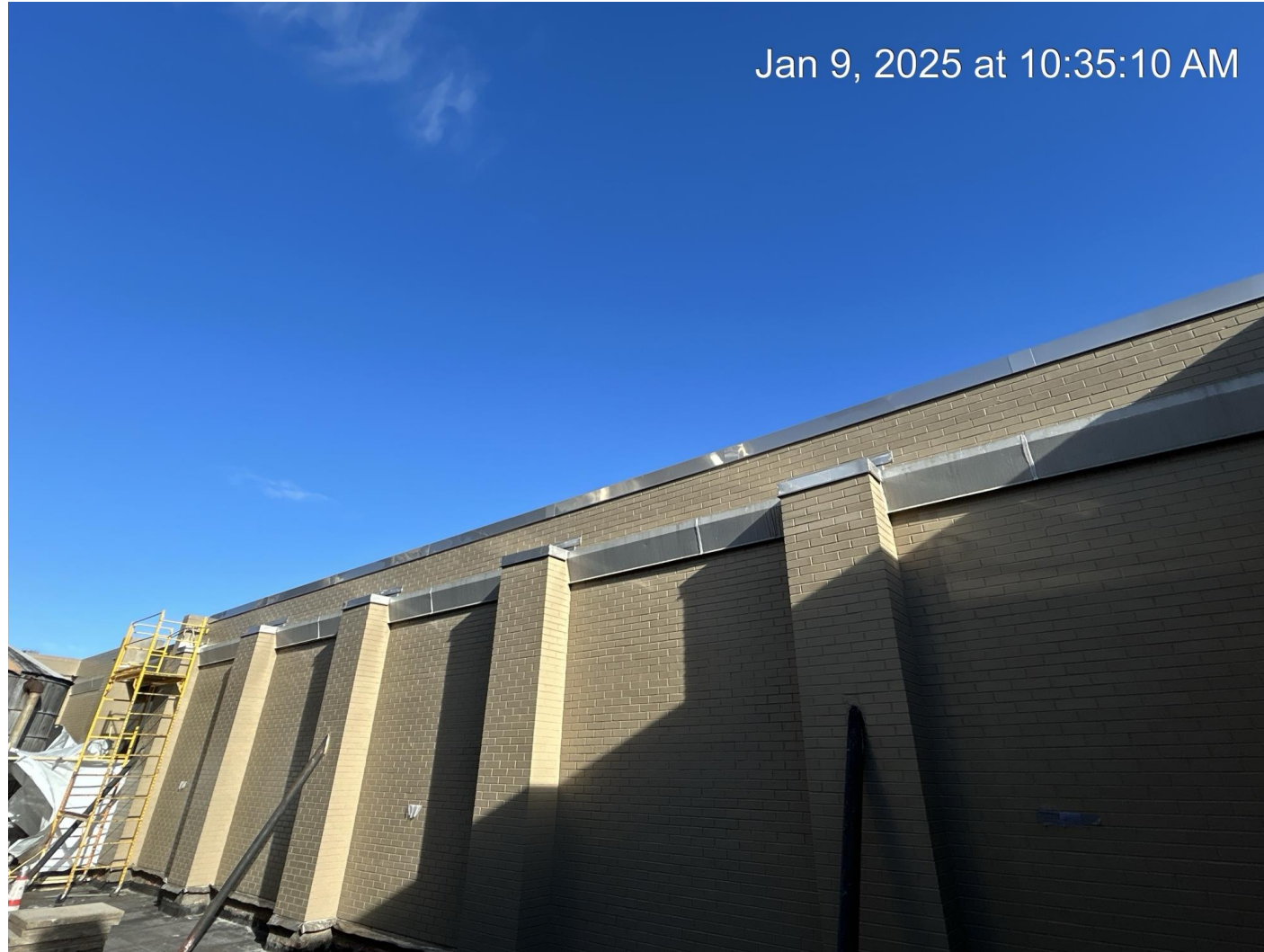
Waterproof coating and new coping installed to the existing Maria's Tower parapet walls.
