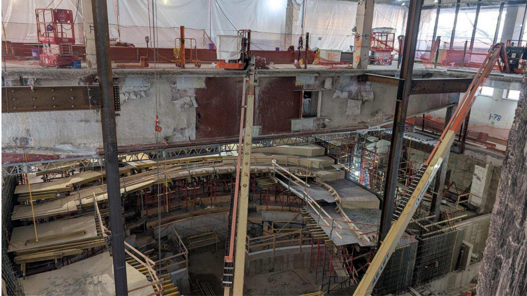
Ongoing structural work in Schimmel Theater, steel and columns are being installed.
